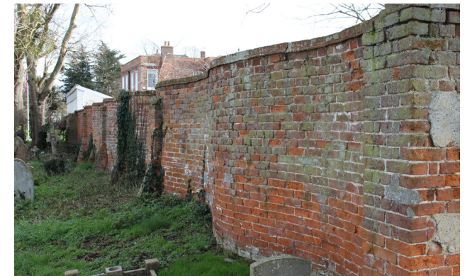
Figure 31 The listed Crinkle-Crankle Wall, which gets its name from its S shape, bendy form
