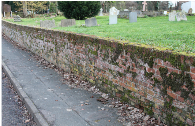
Figure 44 The boundary wall to the Churchyard is in need of maintenance and repair
