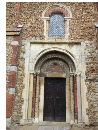
Figure 23 The south doorway of St John the Baptist church showing a variety of materials and detailing
